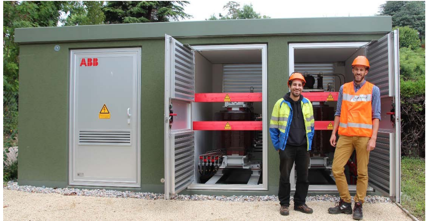
Bruno Gravel and Julien Maret in front of the first Swiss Medium-Voltage Line Voltage Regulator
